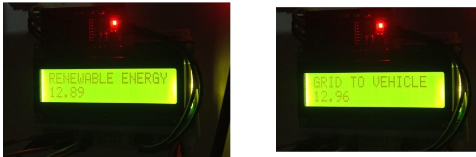
Fig 4: Displaying the battery storage output.
